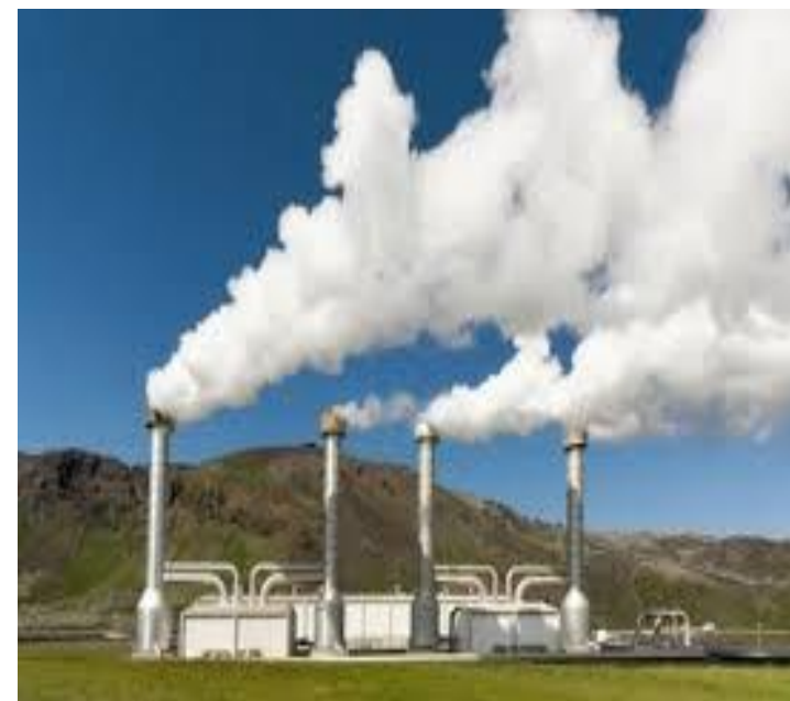
The Kenya's Alkaria Geothermal Plant
